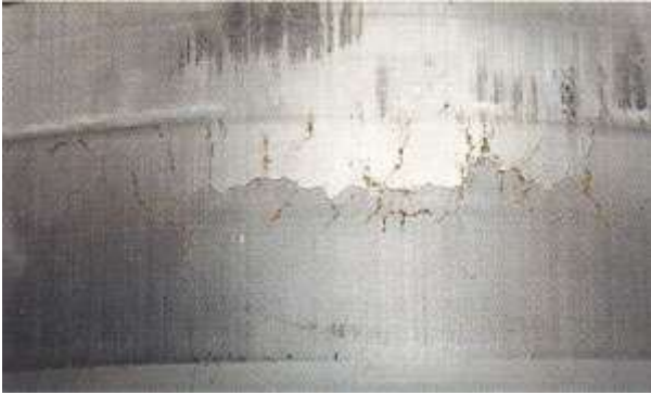
Austenitic stainless steel subject to stress corrosion cracking.
